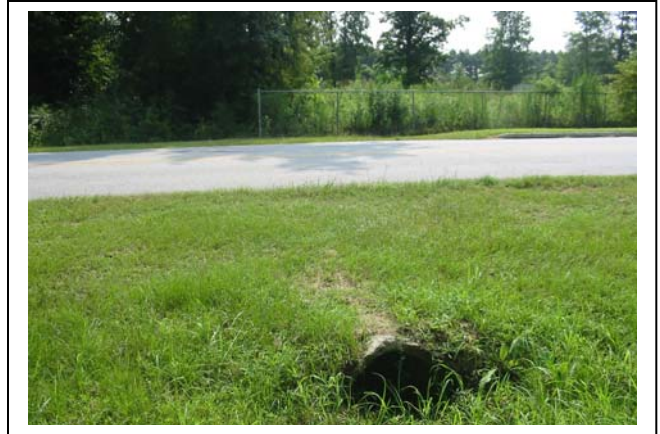
Photo #2: Pipe below Ox Bodies Drive connecting Wetland A to a ditch.
