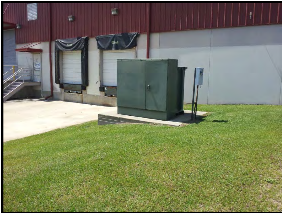
Photograph 10 – Pad mounted transformer and electrical panel (not leaking)
