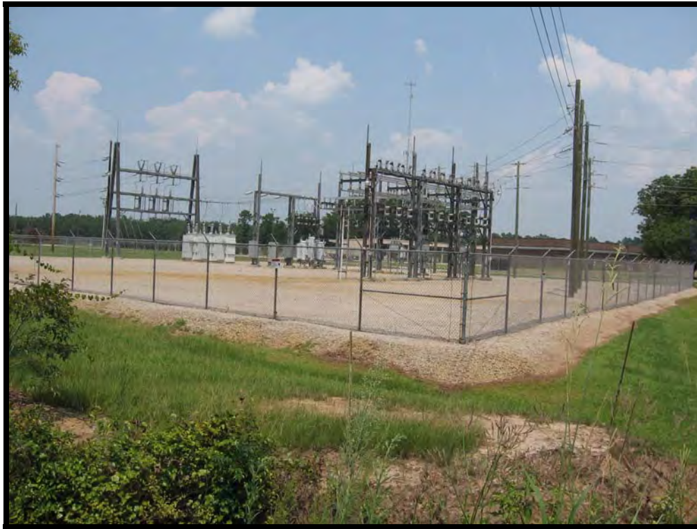
Photograph 33 – Looking north near the Pee Dee Electric Cooperative Sub-Station
