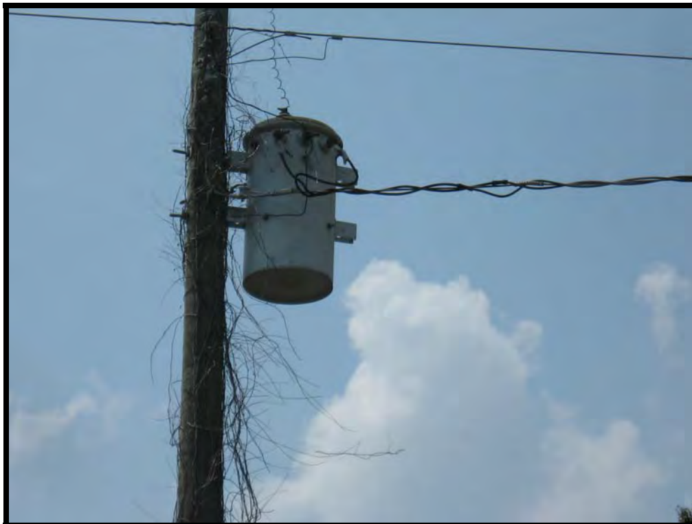
Photograph 42- Looking at existing pole mounted transformer (not leaking)
