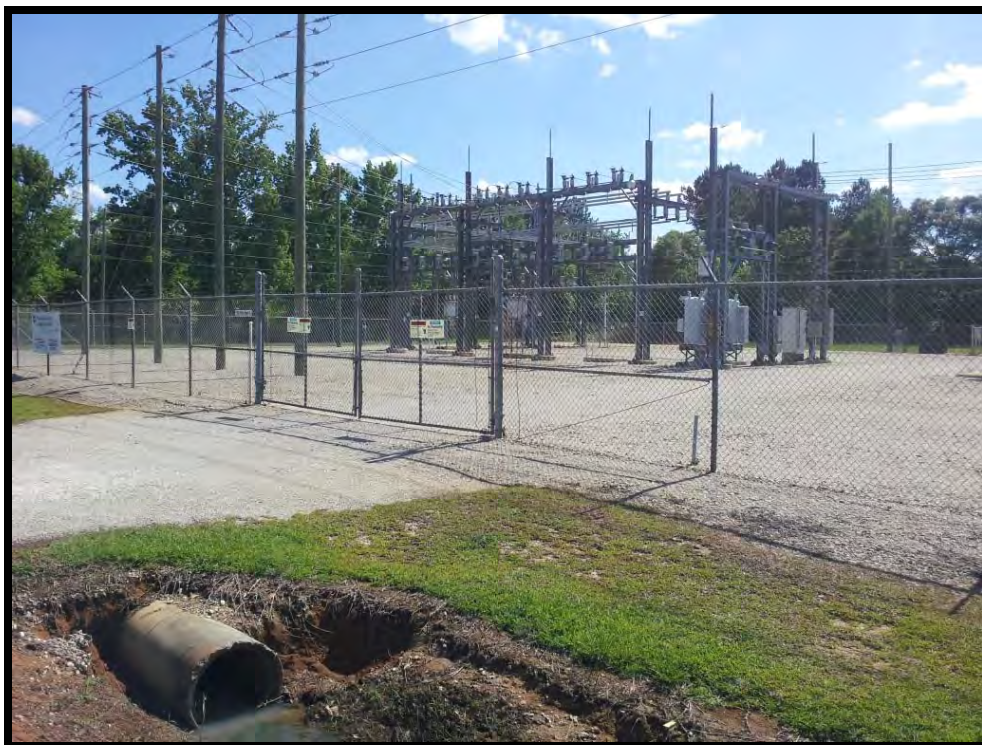
Photograph 20 – Electrical distribution substation located adjacent to the property
