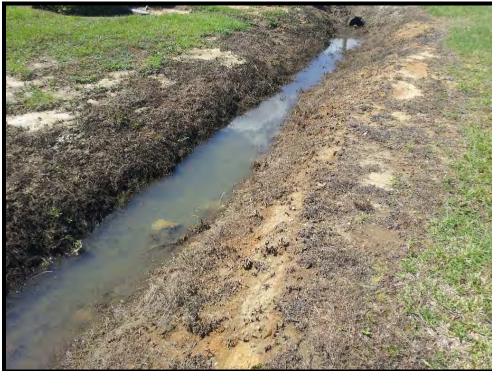
Photograph 18 – Water observed in a roadside ditch along Gurley Road (S-34-681)
